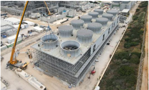
Field Erected Cooling Tower
