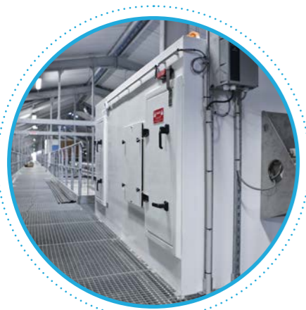
AIR HANDLING UNITS
